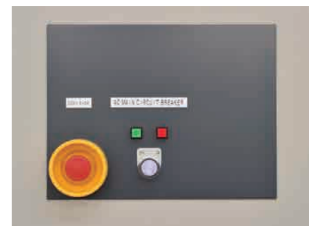
Emergency Stop Button and Circuit Breaker Operation Panel
