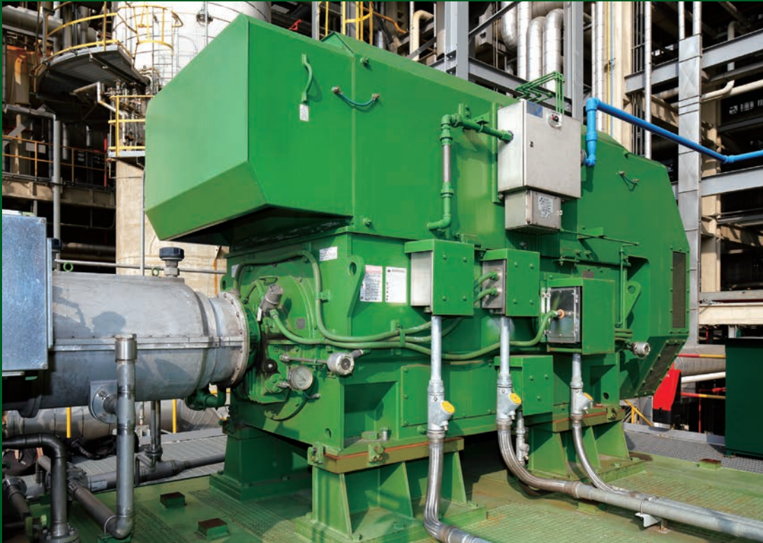
Photos: TMEIC inverter-driven Ex p 4-pole, 1,900kW variable-speed induction motor and compressor
