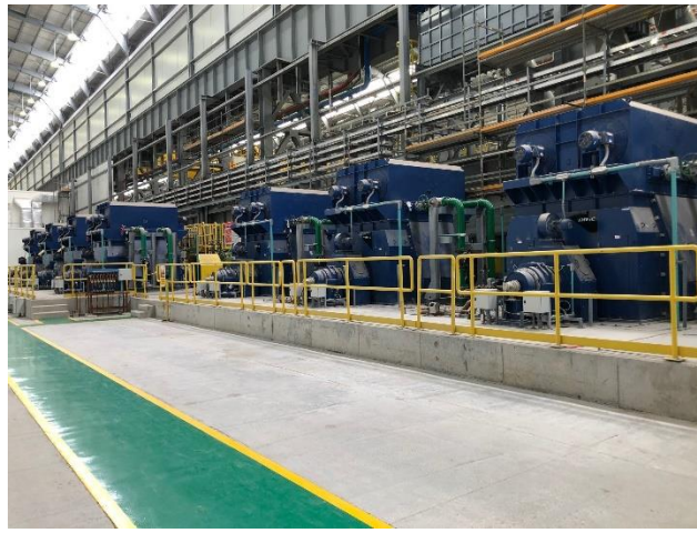
Motors delivered by TMEiC
