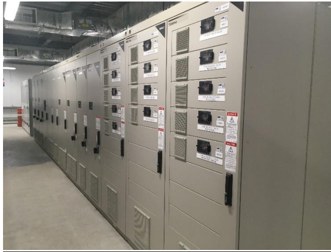
Drive system delivered by TMEiC
